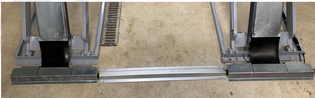
Cover plate at each platform and a cover plate between the platforms.
