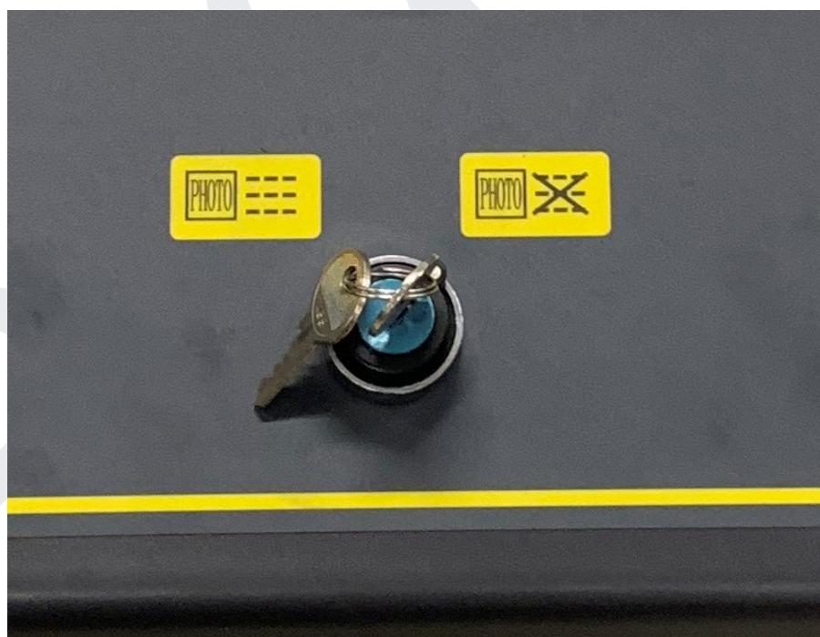
Key switch for Switching the photocell sensor on and off is located on the control box.
